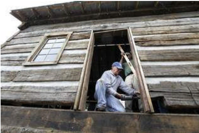
Wilbur Crick, left, and Dave Nachman work on a door frame of an old cabin being restored in Westport. By Michael Clevenger, The Courier-Journal
